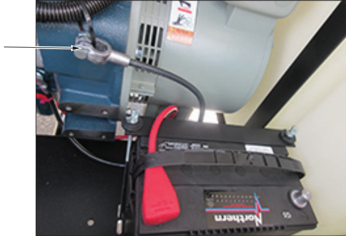
Figure 2 - Negative Battery Cable, Secured Away from Battery
